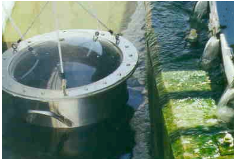
Flux chamber sampling odour from secondary clarifier collection trough
